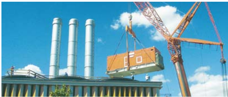
Rooftop installation in a cultural urban environment at Wurzburg, Germany.
